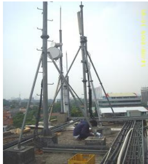
Gambar Rooftop Pole
